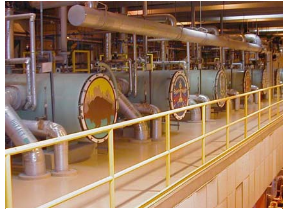
Boilers, located above the engines
