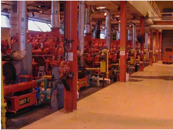
Seven 650-kW Waukesha engines
